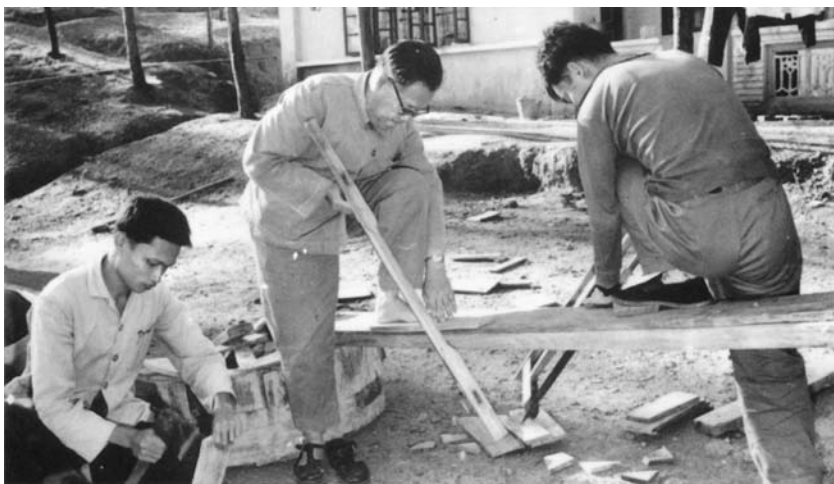
FIGURE 12. Pu Zhelong’s wristwatch clearly marked him as a man of position, but he was not above engaging in manual labor in this photograph of construction at Big Sand’s new bacterial fertilizer factory (c. 1975). Reproduced from Gu Dexiang, ed., Pu Zhelong jinian yingji (Pu Zhelong memorial album), 2002, 25.
