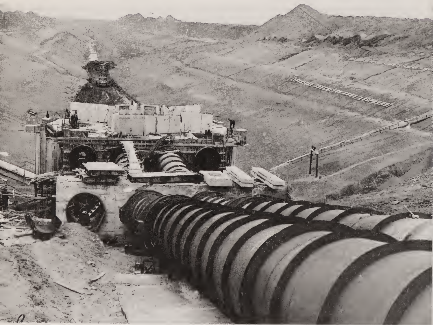
The laying of pipes to convey water from the upper Irtysh River to Karaganda in the dry steppes of northern Kazakhstan (SCR)
