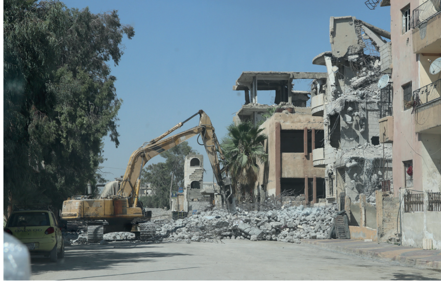
Many buildings in Raqqa need to be demolished and rebuilt
