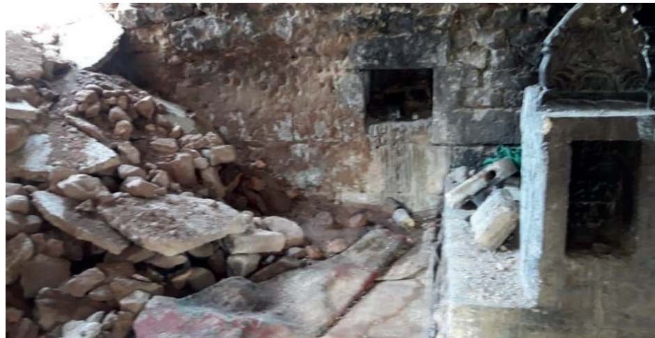
The interior of the Sheikh Humayd shrine in Afrin following the partial collapse of its roof
