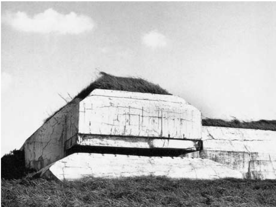
Two types of observation posts: with curved sections and with flattened angles
